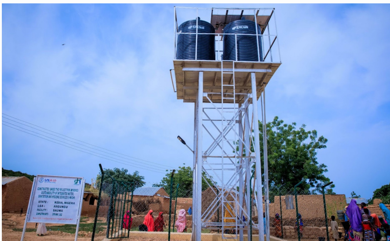
Figure 6: Showing a newly constructed 12,000 ltr capacity solar-powered borehole in Bayan saula community in Sauwa ward, Argungu LG, Kebbi State.
