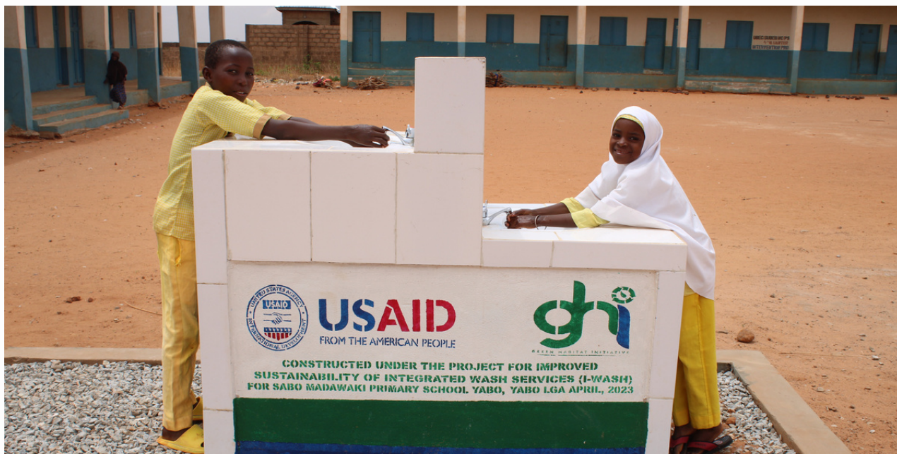
Figure 7: A newly constructed handwashing in Madawaki Primary School in Yabo LGA, Sokoto State.
